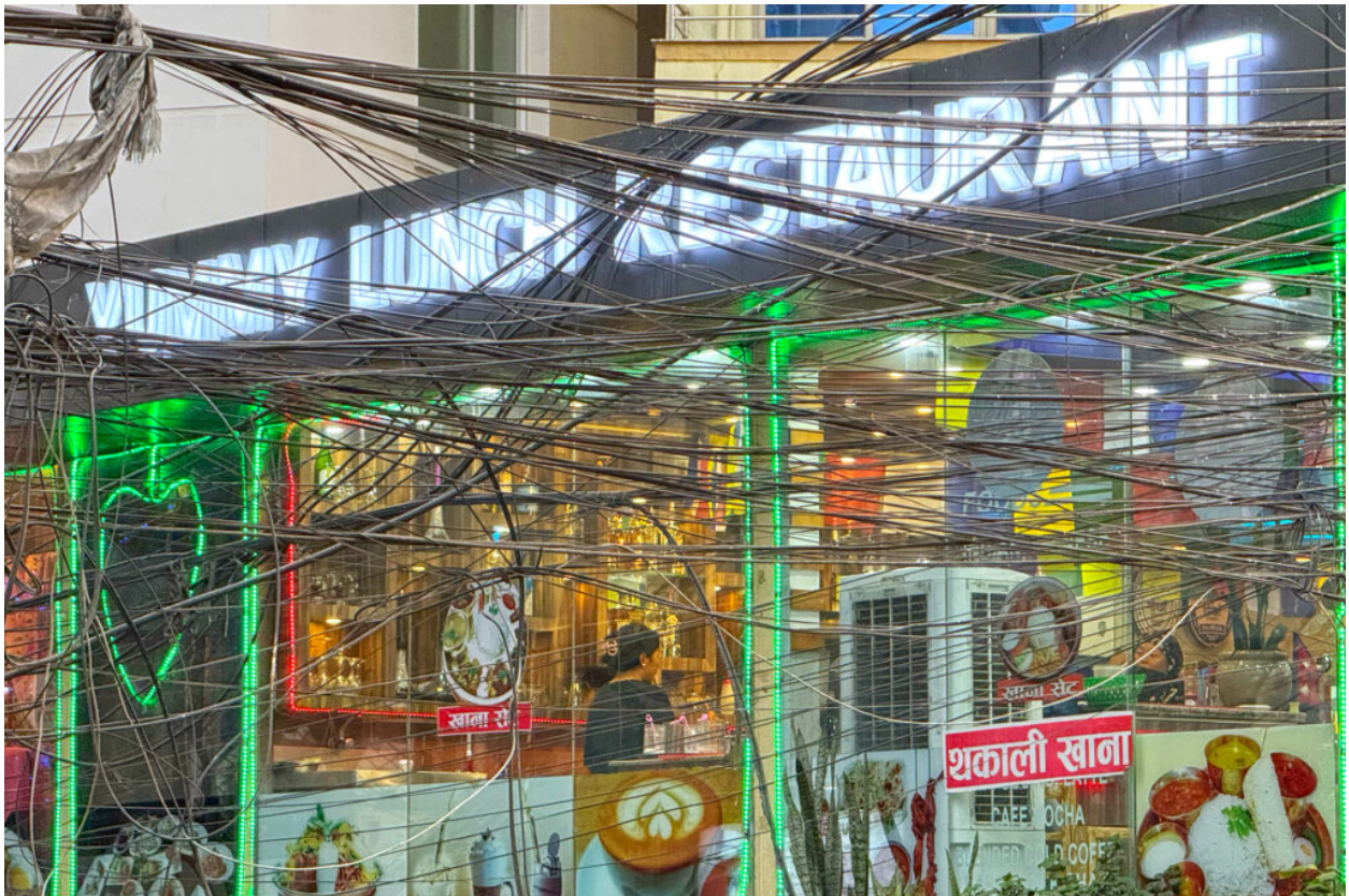
Electricians nightmare (image by Mike Watson)
